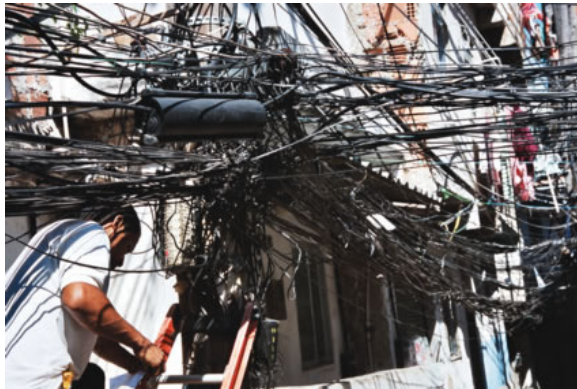
Illegal power wires also known as “gatos” attach to formal wires to provide residents with free power.
